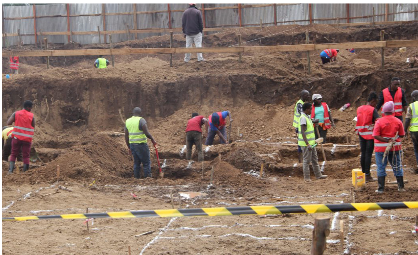
Affordable Housing Program: Workers digging foundation of the affordable house units in Nanyuki Municipality
