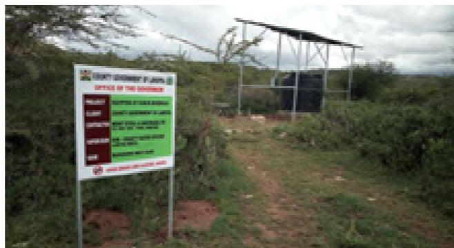
Appendix 4: Ongoing solar equipping of Ethi community borehole
