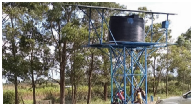
Appendix 13: Solar Panels, Tank, Pump controller and CWPat Machunguru B/Hole
