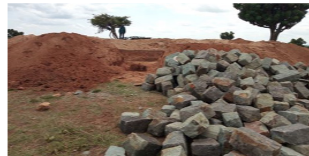
Appendix 9: Foundation excavation for the 225M3 masonry tank and materials for Osirwa W/P
